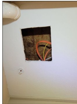
Opening in service panel room near garage
