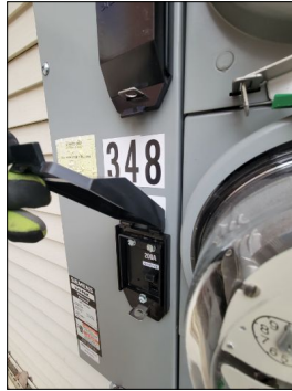
Disconnect at meter near garage
