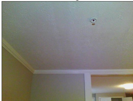
Indicated previous repair dry, ceiling in primary bedroom
