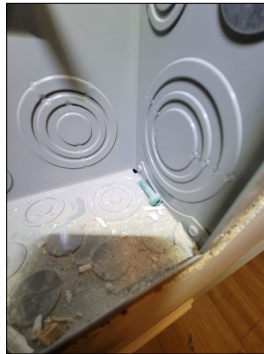
Bonding screw not attached, required for main panels (this is not a remote distribution panel)
