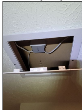
Garage, panel to access electrical junction box
