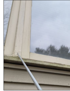
Some wood rot, front
