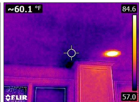
Indicates missing insulation in kitchen ceiling at front wall
