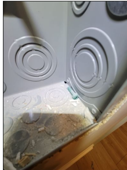
Bonding screw not attached, required for main panels (this is not a remote distribution panel)
