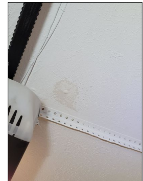
Currently dry, garage
