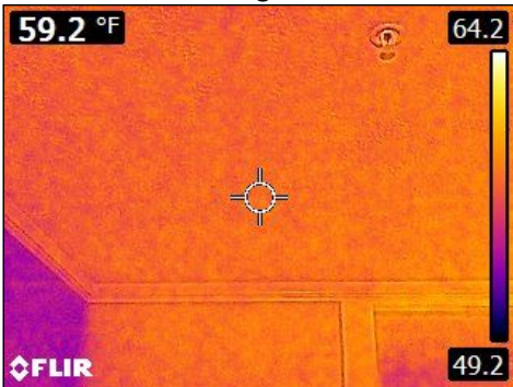
Indicated previous repair dry, ceiling in primary bedroom
