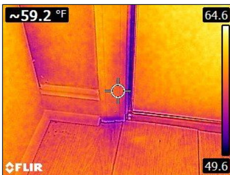
Indicates some cool air entering entry door (storm door at top of stairs needs new weatherstripping/adjustment)
