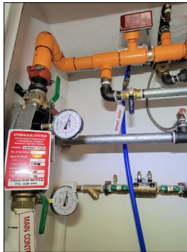
Above water heater in primary bedroom closet
