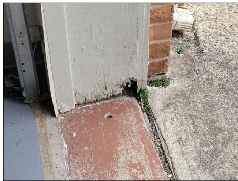
Some wood rot
