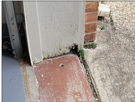
Some wood rot
