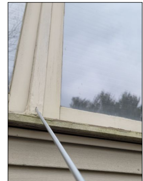
Some wood rot, front
