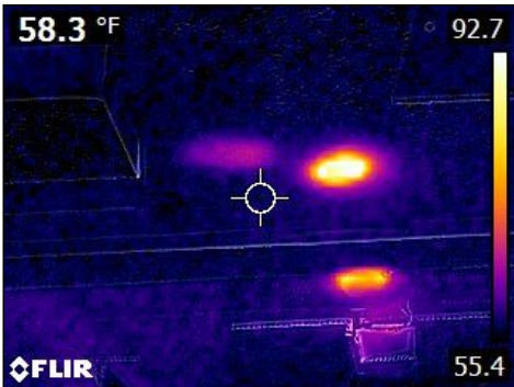
Indicates a bit of heat in garage ceiling (likely the junction box for the recessed light nearby), okay of contained in box
