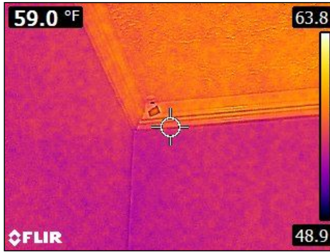
Indicates dry repair, primary bedroom ceiling at corner
