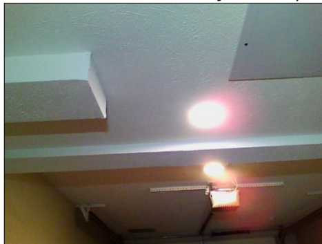
Indicates a bit of heat in garage ceiling (likely the junction box for the recessed light nearby), okay of contained in box
